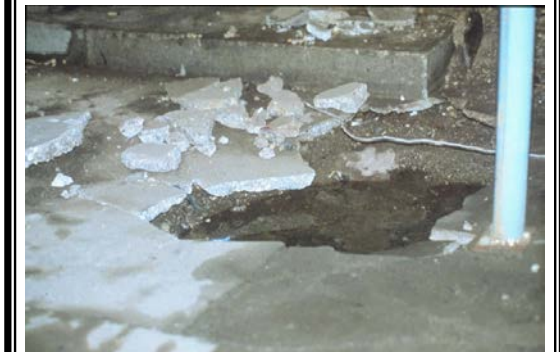
This basement floor broke due to hydrostatic pressure
