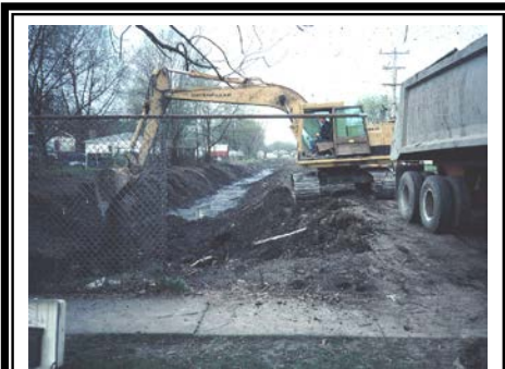
Some channel improvements can be very damaging to the environment and may pass a flooding problem onto downstream properties.
