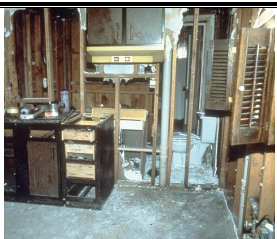
Effects of soaking on walls, floors and cabinets.
