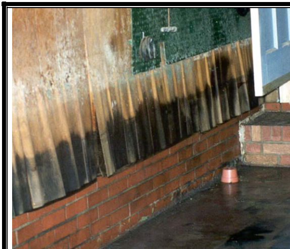
Soaking delaminates plywood and the wicking effect means that damage will be higher than the flood level.
