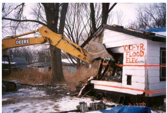
This home in Lake County was not worth relocating, so it was acquired and demolished by the County. The site is now open space.
