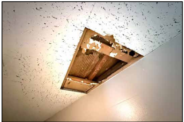
22. Missing 1' x 1' tongue and groove ceiling tiles and exposed damaged drywall above former X-ray room.
