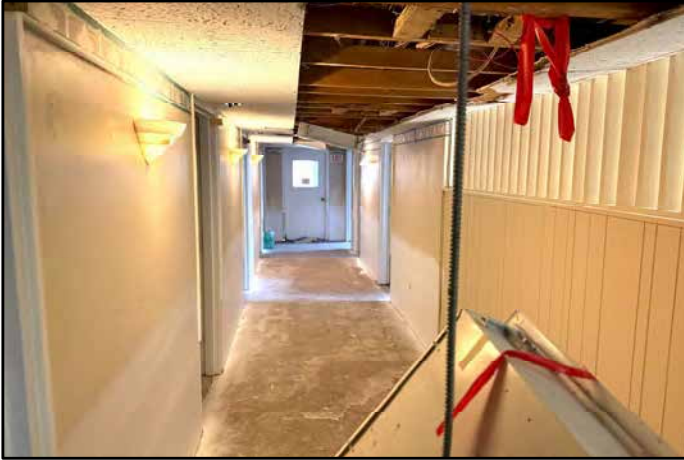
25. Basement hallway inside subject building; observe removed floor tiles.
