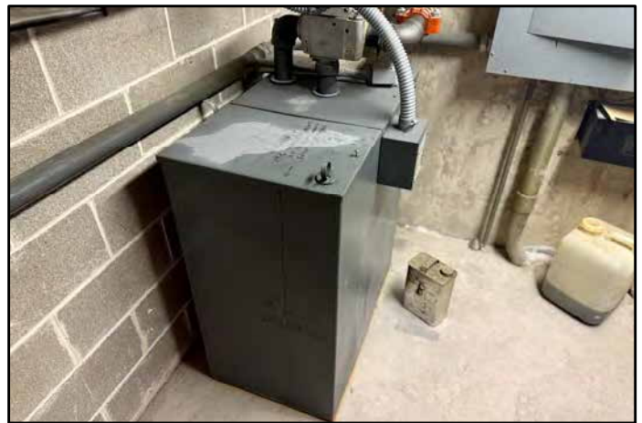
30. Hydraulic oil reservoir tank for elevator inside basement.
