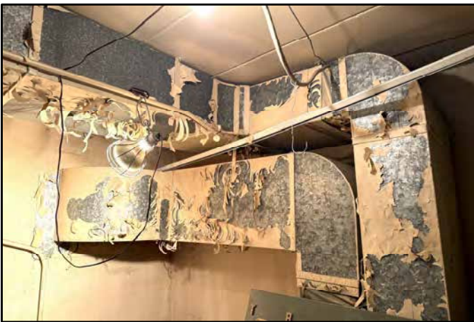
27. Peeling paint on ductwork inside basement; isolated.
