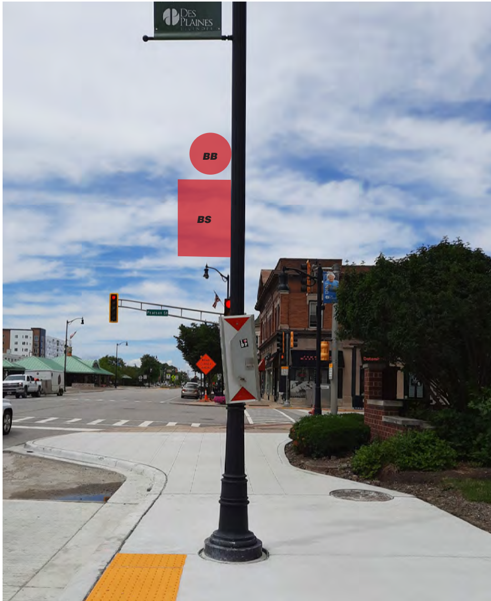
New sign panels and mounting hardware replace existing Pace bus stop sign on light post.
