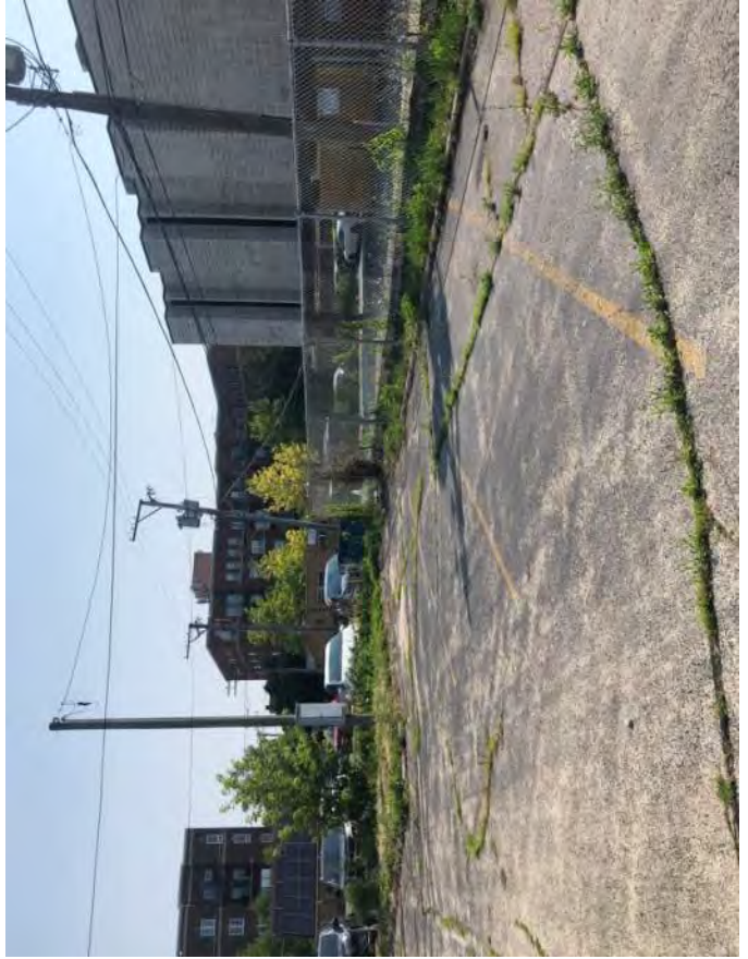
View of existing parking lot facing alley to northeast; degraded pavement
