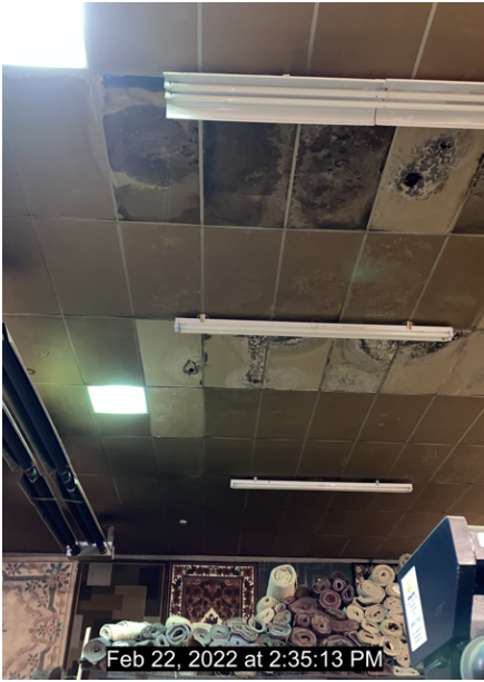
Mold from roof disrepair and debris inside building
