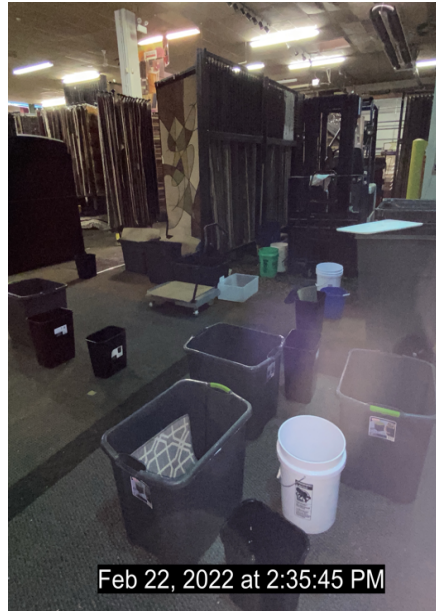
Pool collecting water from leaking roof
