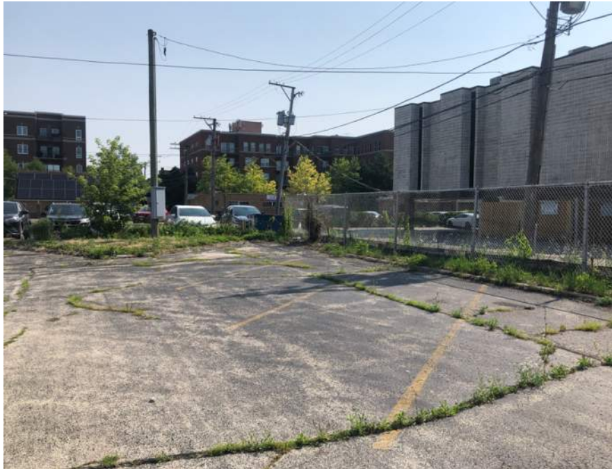
View of existing parking lot facing alley to northeast; degraded pavement
