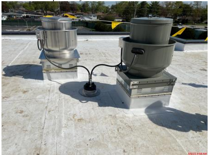
Exhaust fans on roof, wired into pipe portal.
