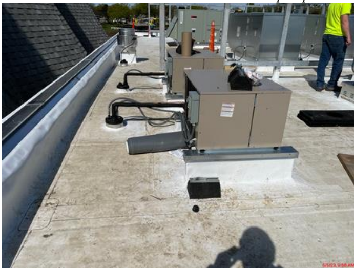
Condenser units for cooler and freezer.
