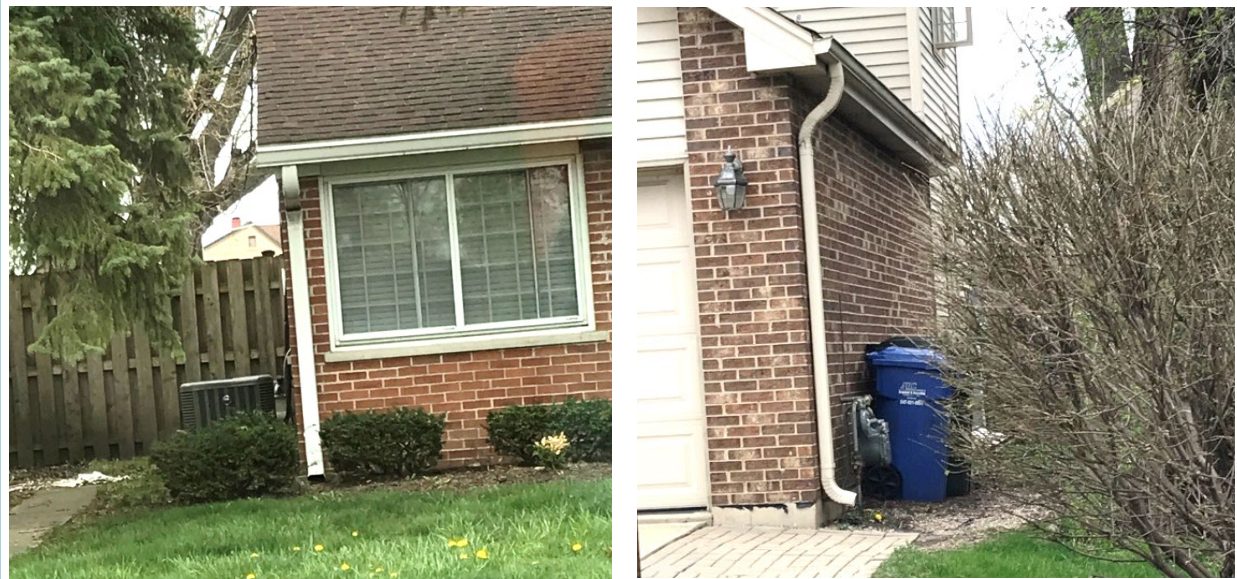
Figure 25. Typical downspouts in Repetitive Loss Area 10. As shown above, many of the downspouts within Repetitive Loss Area 10 were not extended. The majority of structures in this area do not have basements; therefore, seepage and continually running sump pumps may not be an issue.
