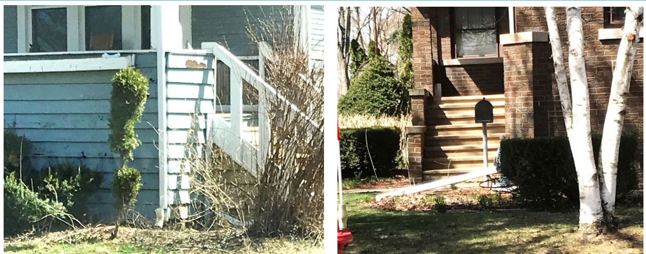
Figure 13. Downspouts in Repetitive Loss Area 4. Downspouts in Repetitive Loss Area 4. The image on the left shows a downspout that has been extended away from the structure and the image on the right shows one that has not been extended.
